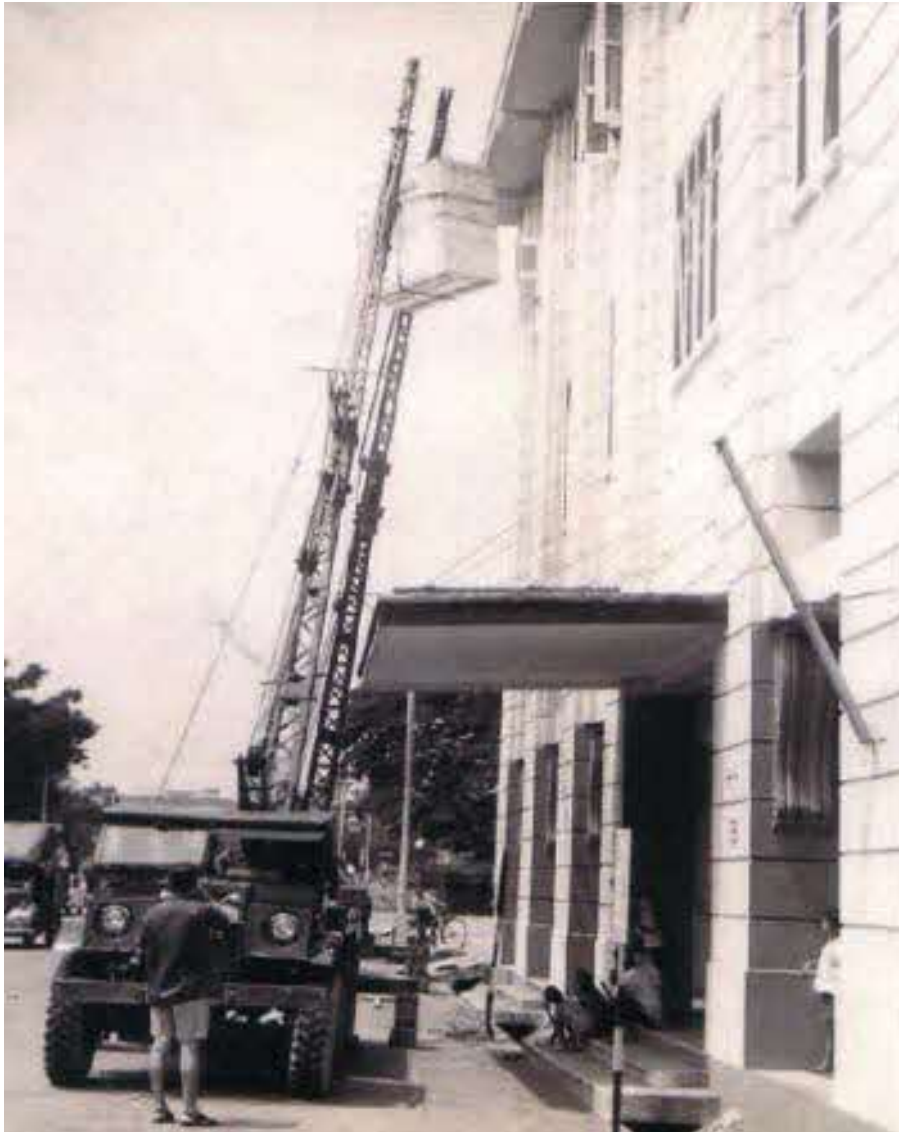
◀ Parts of the IBM1401 Data Processing System being lifted through the window at the CPF Board headquarters at 79 Anson Road. (Source: CPF Board)
